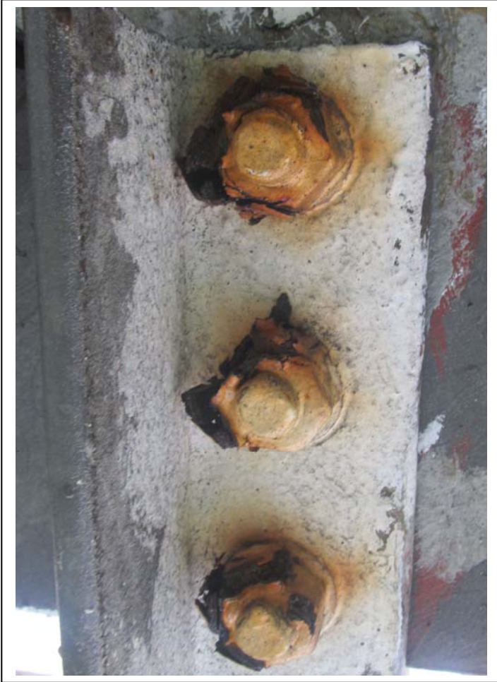
Photo No. 21 (Before)
