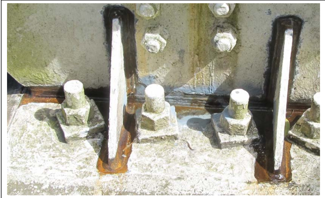
Photo No. 34 (Before)
