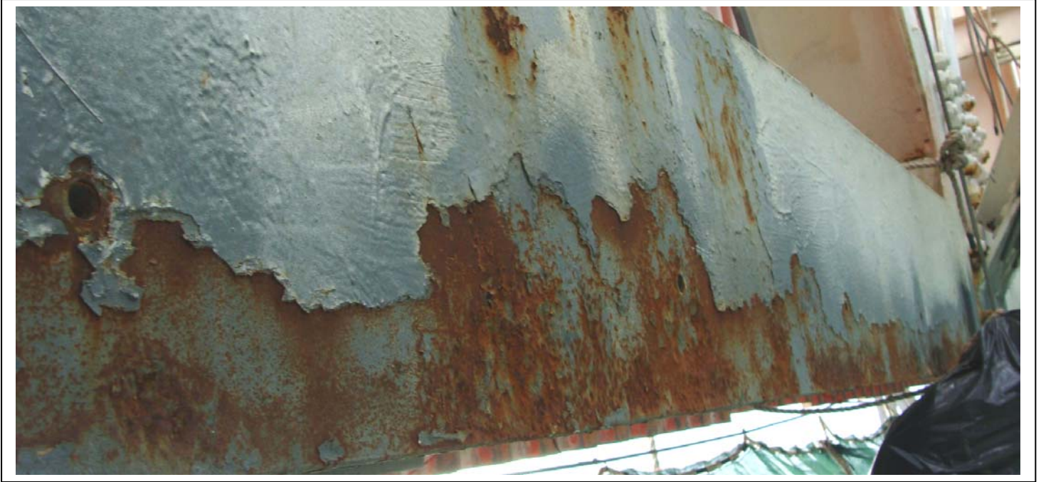
Photo No. 10 (Before)
