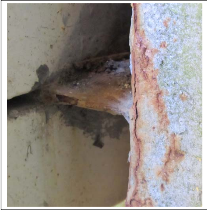
Photo No. 25 (Before)
