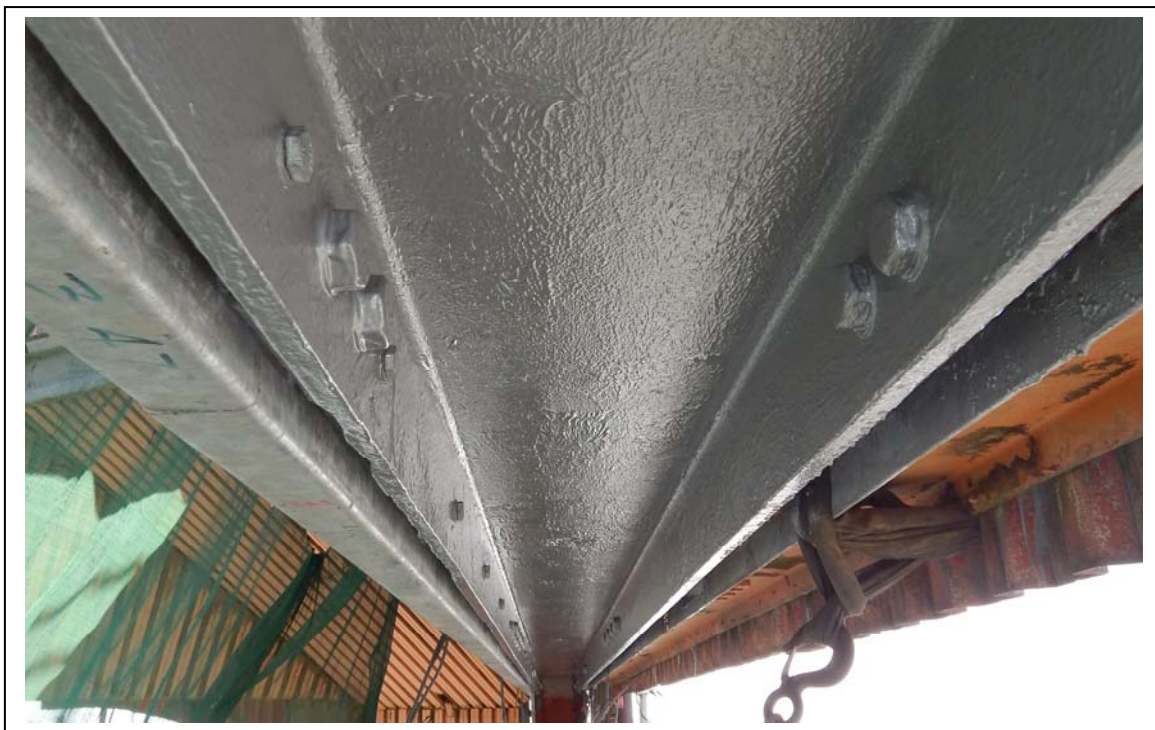
Photo No. 13 (After)
