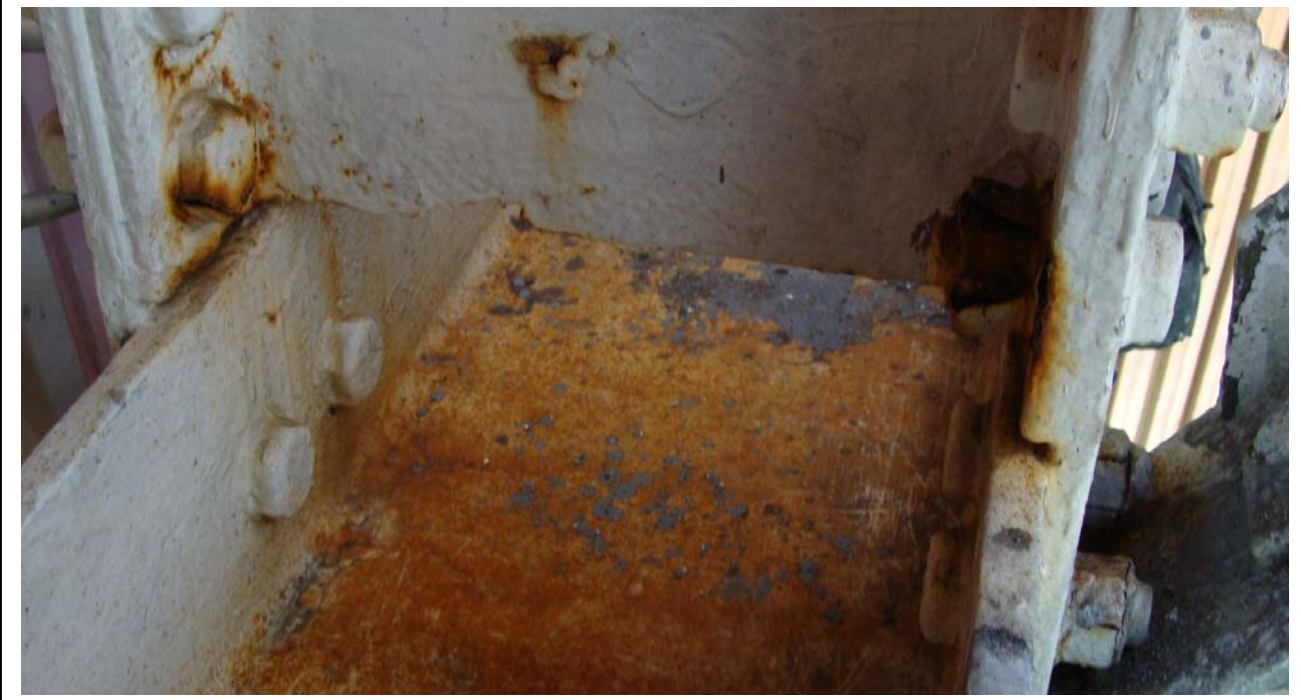
Photo No. 19 (Before)
