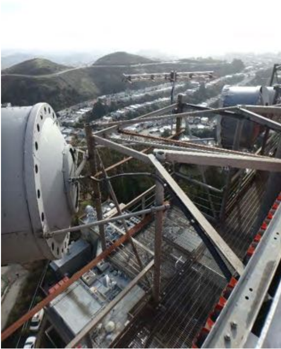
Minor Rust Throughout Mounts
