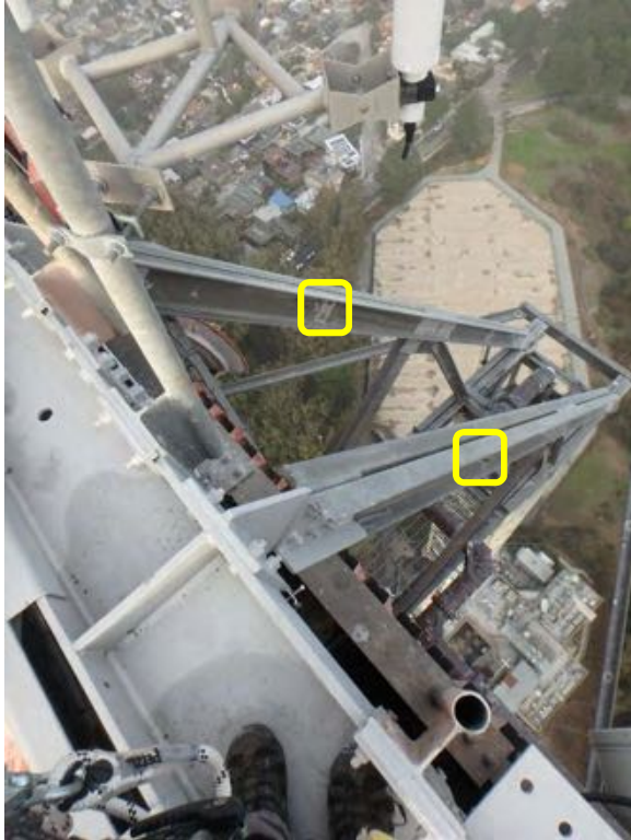
Minor Rust on Multiple Bolts Throughout Mount
