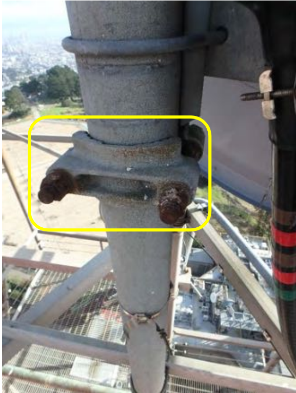
Minor Rust on Multiple Bolts Throughout Mount
