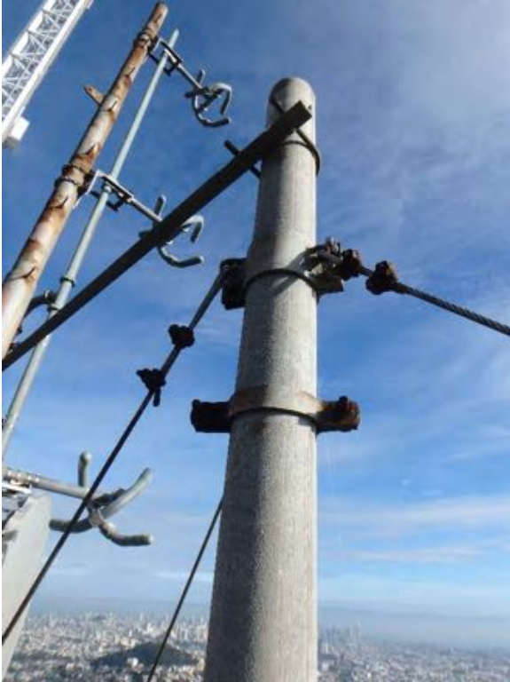
Minor Rust on Multiple Bolts Throughout Mount
